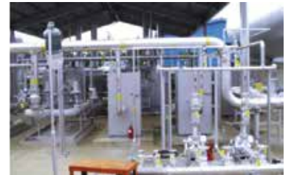
LPG vaporization and mixed equipment
