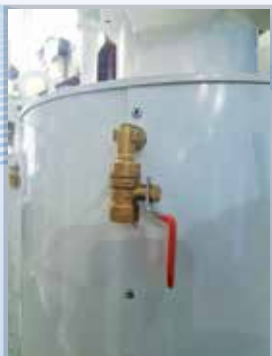
Water Overflow Valve (Prevent the Water Evaporation)
