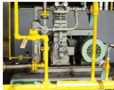
Ammonia Unloading Compressor
