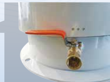
Water Drain Valve
