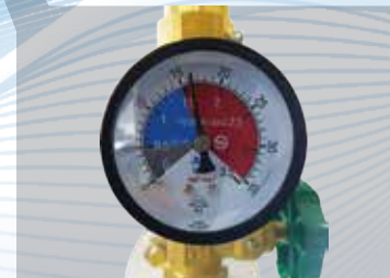
Gas Pressure Gauge
