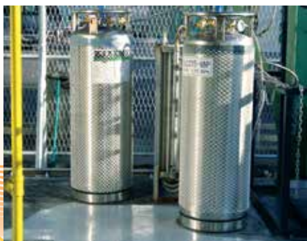
N 2 Purge System
