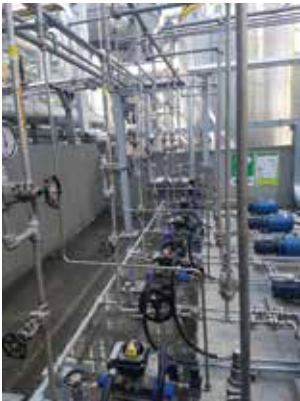
Aqueous Ammonia Supply System
