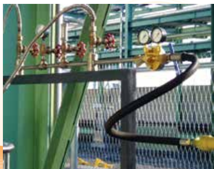
N 2 Purge System
