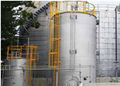
Aqueous Ammonia Storage Tank
